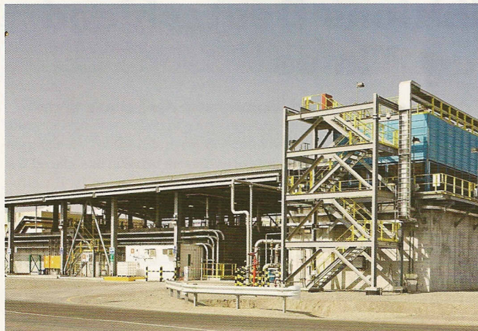
Fives Solios water-cooling plant at Sohar Aluminium
